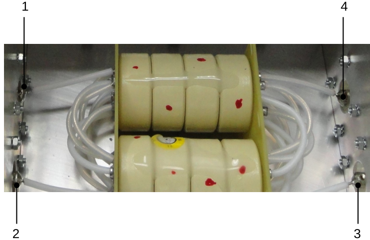
Figure 5. A photograph of the high-power 4-ports transformer. A fan is used to continuously cool down the ferrite rings and it is located on the lid of the aluminum box. The ferrite cores and the winding can be clearly distinguished. 1: port (1); 2: port (2); 3: port (3); 4: port (4). Coaxial cables (i.e., with inner and outer conductors) are used as winding wires. A closer look at port-1 shows the mounting of the coaxial winding to a ‘7/16’ connector. The ports of the transformer are marked in figure 1.
